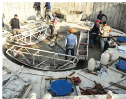
Seismic isolators at the new site
